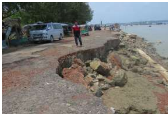
Fig. 4: Damaged road at Raychata of Banshkhali.
